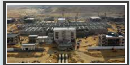
Tertiary Treatment Plant
