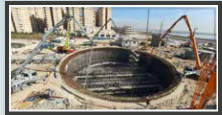
Water Pumping Station from Western TP
